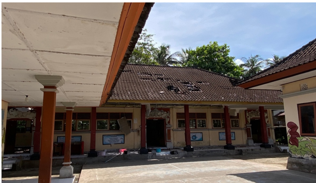
Figure 2. Classroom building that suffered severe damage to the roof in Karangasem Regency
